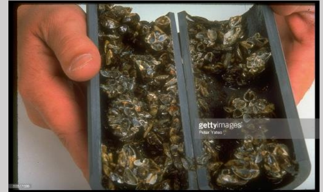
Clogged Water Pipe
