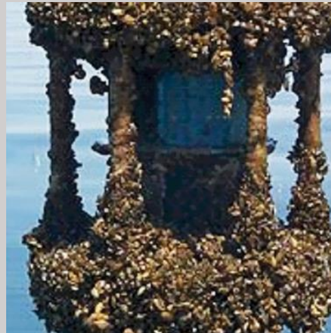
Power Plant Water Intake
